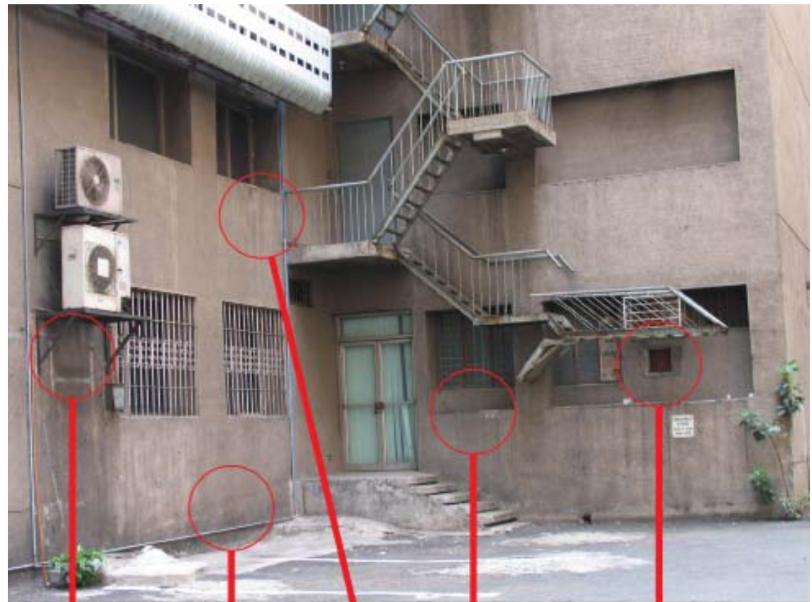
Dirt and water from A/C system
